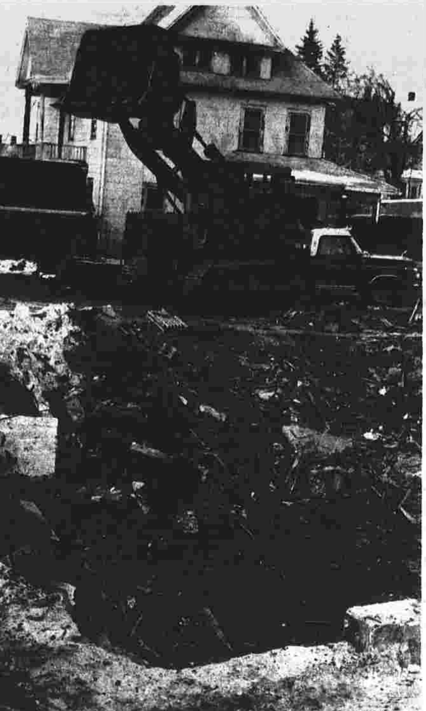
Building leveled Workers have leveled the remains of a building, formerly 451-459 Main Street, which was destroyed in a Dec. 6 fire. Construction crews have also begun filling the hole left in its basement, where officials have determined the fire started. The building had housed the Manchester Safe and Lock Co. and the Little House of Foxes, a former massage parlor. (Herald photo by Pinto)
